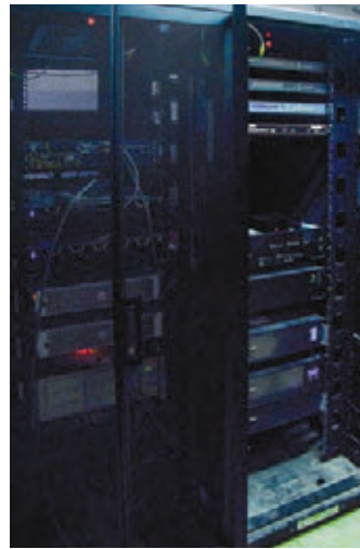
The rear second-level room hosts multichannel amplifiers, audio distributors and a DP-SP3 processor
